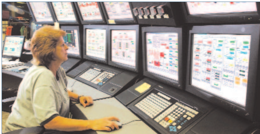
Cheryl Barnett uses state-of-the-art equipment to monitor the pollution control equipment and electric generation at A.B. Brown.
